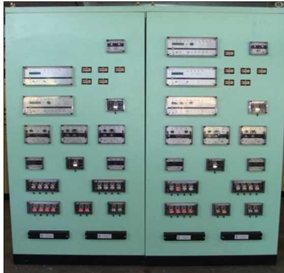
Figure 8 Control and Relay panel with Static Relays
