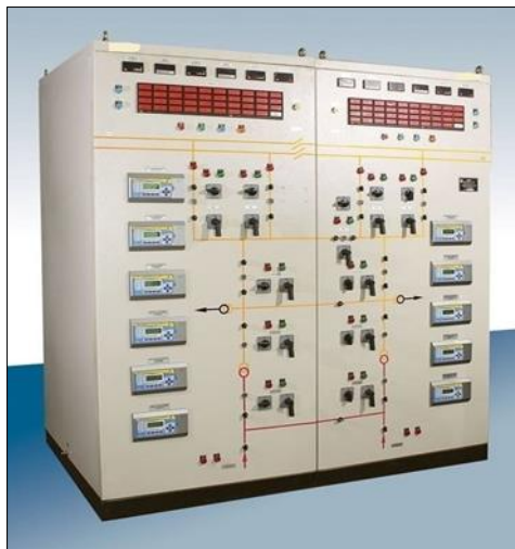
Figure 10 Control and Relay panel with Numerical Relays
