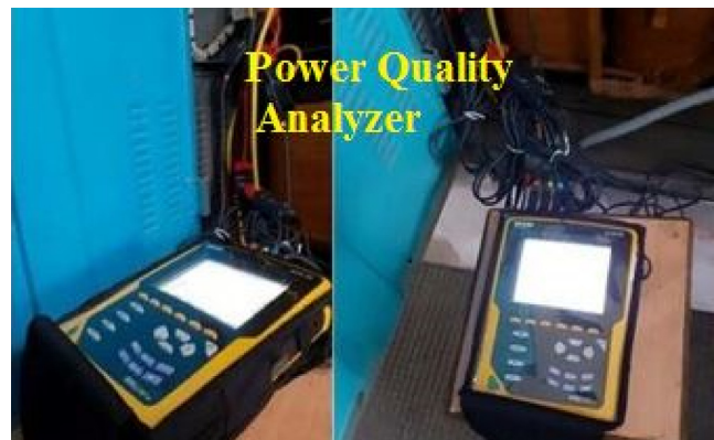
Fig. 3 Power quality analyzer.
